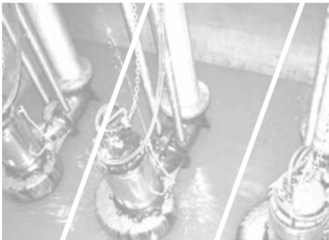
Wastewater Transport and Treatment
